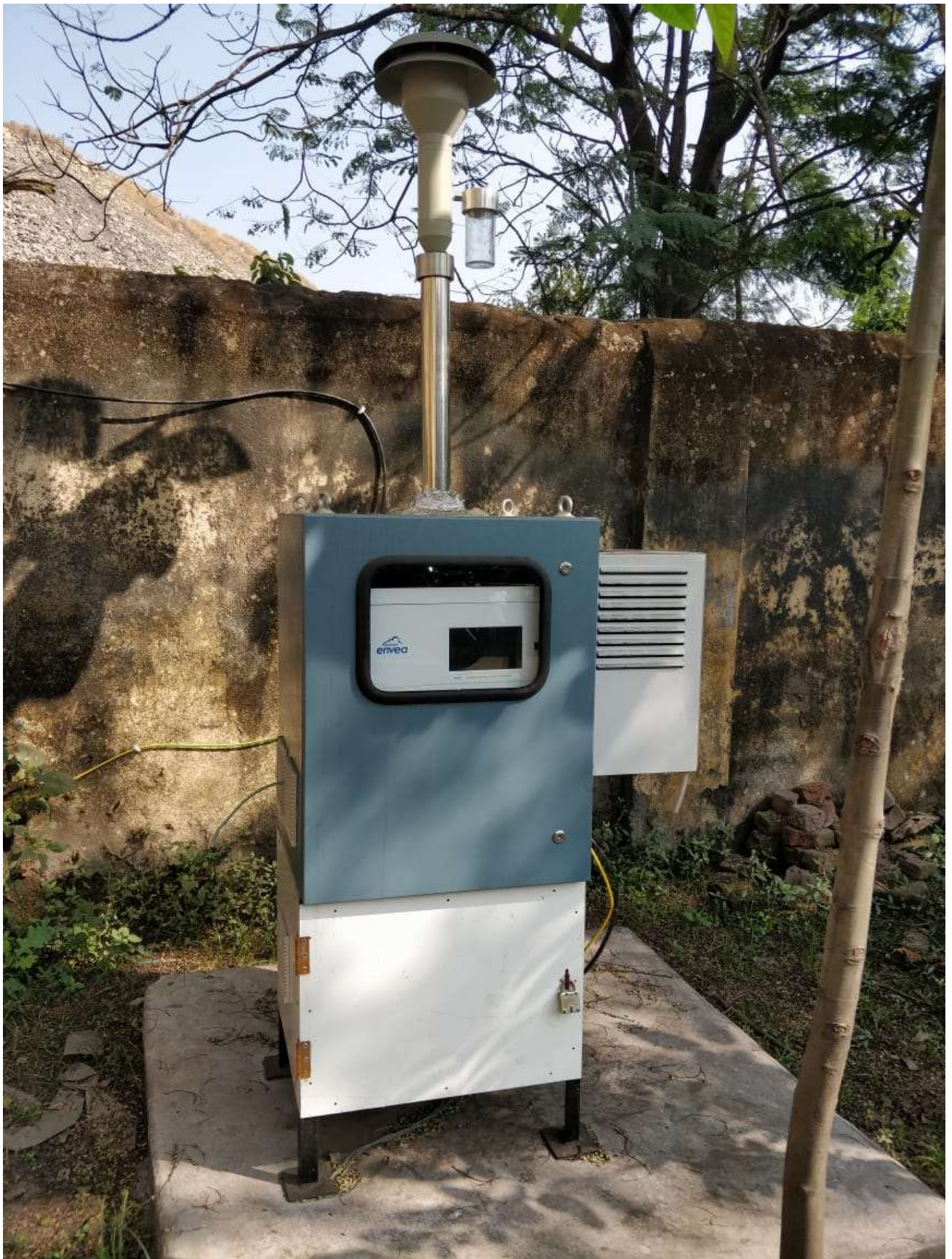
Picture 14- PM 10 Analyser Installed
