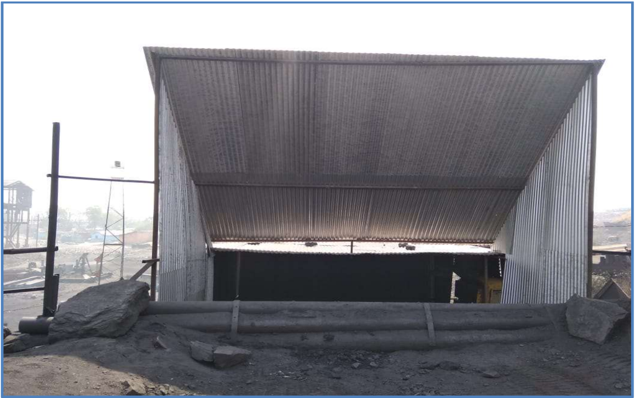
Picture 7 – Enclosed Coal Handling Plant
