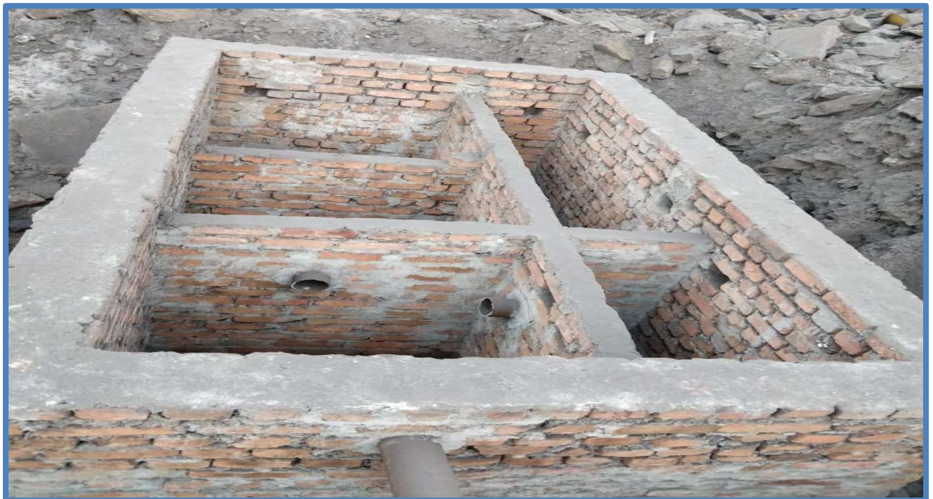
Picture 10 – Oil & Grease Trap
